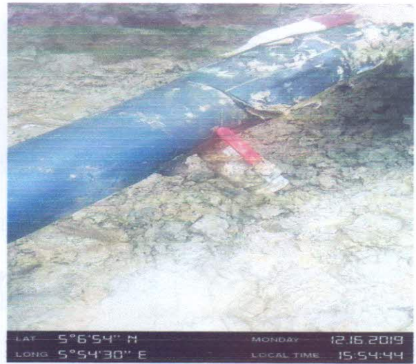
Pic 2: After excavation 3" Ball valve found.
